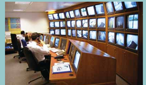
Security Systems / Control Room
