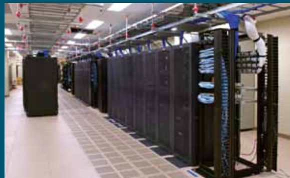
Offices, Workstation and Lan Servers
